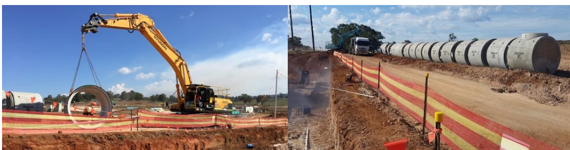
Interim Operating Pump Station
