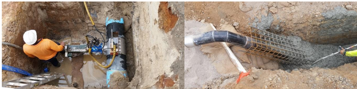
Water Main Lead-In
